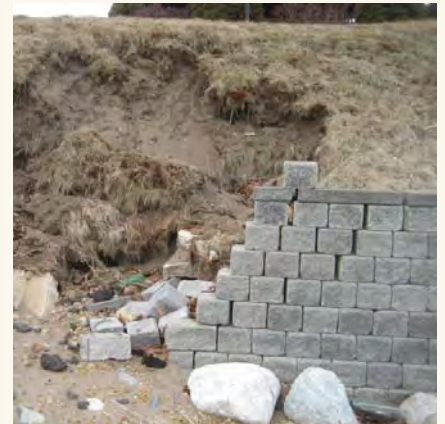
Example of Dry Stacked Block Seawall Failure. Avoid using block walls in high wave and ice scour prone areas
